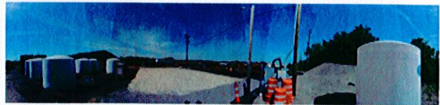
Image 3 - View from Left to Right: Foreman House (not constructed at time of photo); 10 x 15 Steel Tanks (8,400 Gallons); 10 x 10 Poly Tanks (8,100 Gallons); In-Process Tanks (20,000 Gallons)
