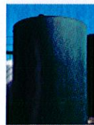
10 x 15 Steel Tanks (8,400 Gallons)
