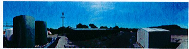
Image 1 - View from Left to Right: 10 x 10 Poly Tanks (8,100 Gallons); 10 x 15 Steel Tanks (8,400 Gallons); Raw Storage Tanks (20,000 Gallons); Shed
